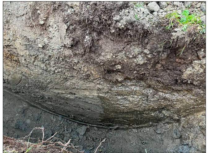
Photo 4: TP-2 conditions. Note seepage along topsoil-GMD boundary.
